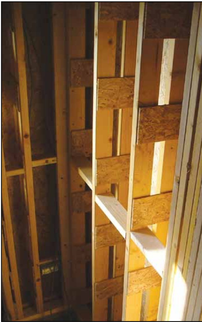
Figure 17: Twin-wall construction with OSB gussets prior to filling with insulant (image: courtesy of Williams Homes)
