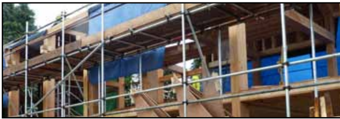
Figure 10: Ty Unnos portal frames erected at Blaengors, Carmarthenshire (image: courtesy of Coed Cymru)
