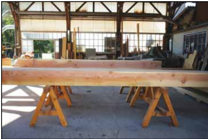
Figure 7: Douglas fir posts and beams being prepared in a local workshop in France
