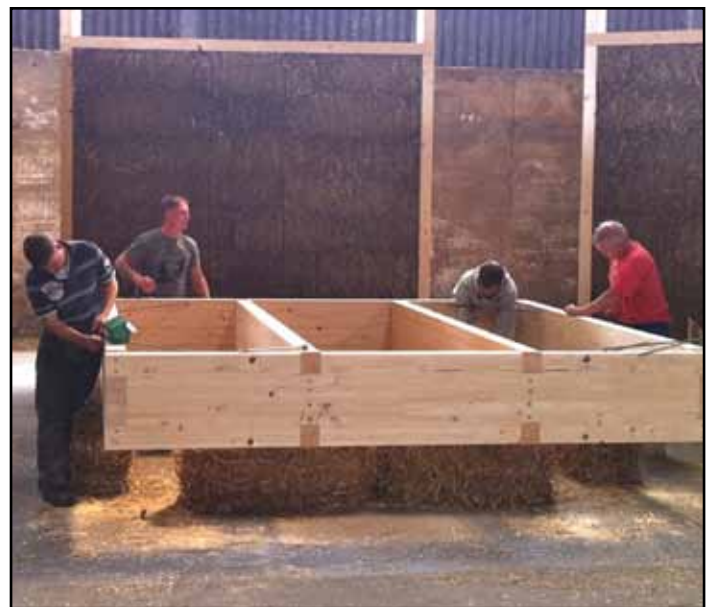
Figure 26: A Modcell cassette being fabricated in a 'flying factory' (image: courtesy of Craig White)
